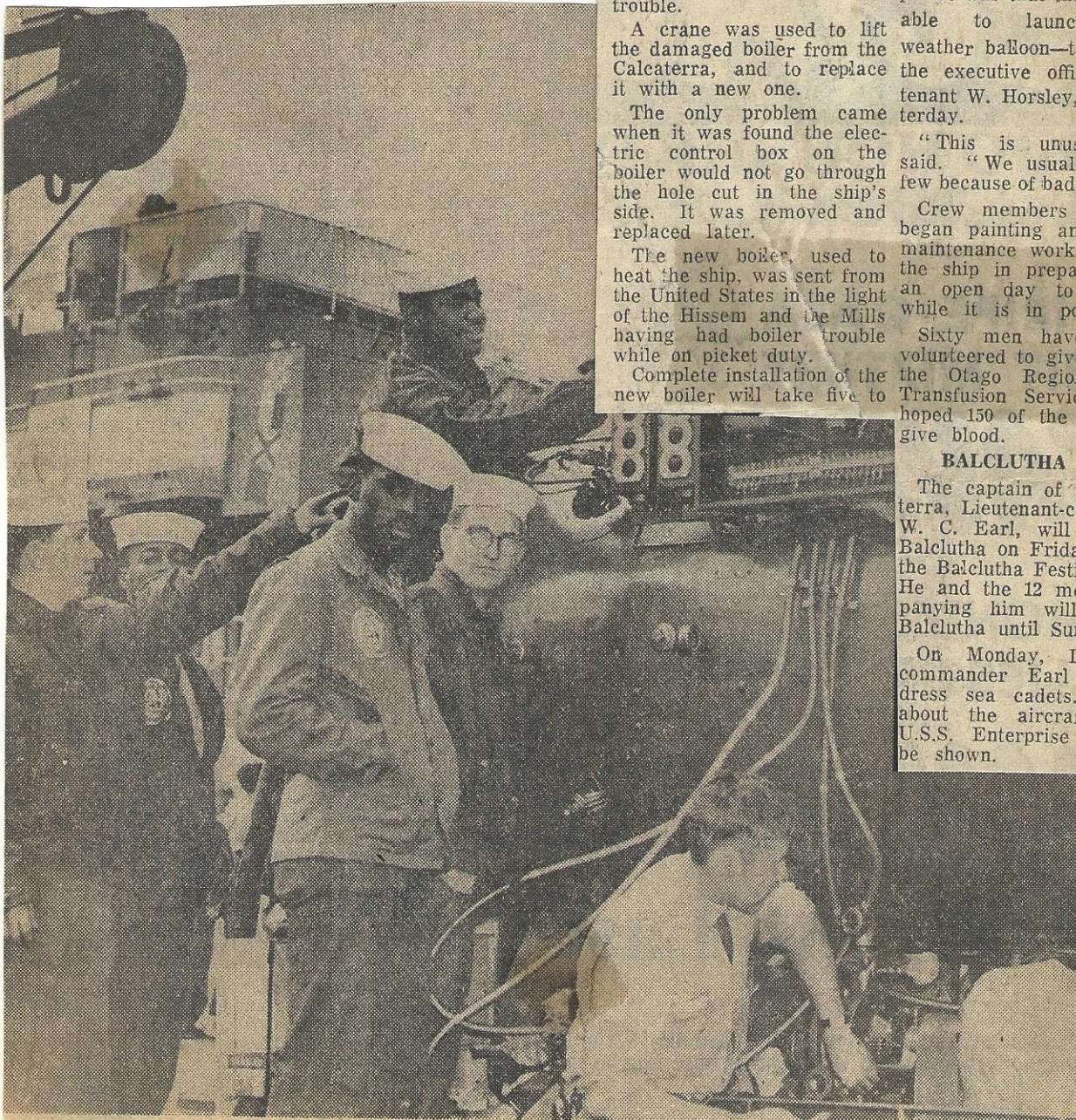
CREW MEMBERS of the U.S.S. Calcaterra take a look at the new boiler which will replace the one damaged while the weather picket ship was on ocean station. The boiler was manoeuvred into position this morning through a hole cut on the port side of the Calcaterra.
